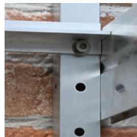
Bolt sits below staging rail
