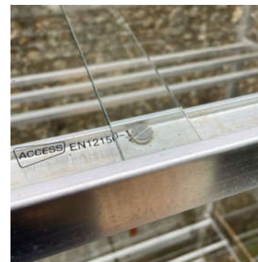
Roof glass overlapping
