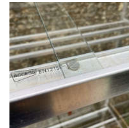
Roof glass overlapping
