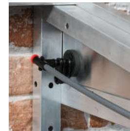
Inlet and link pipe
