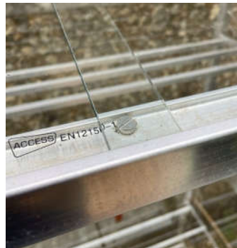
Roof glass overlapping
