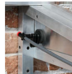
Inlet and link pipe
