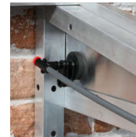
Inlet and link pipe
