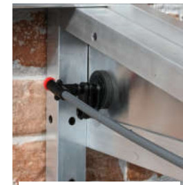
Inlet and link pipe
