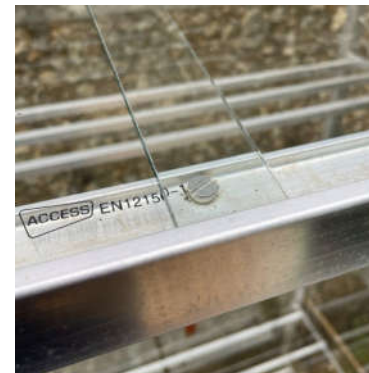
Roof glass overlapping
