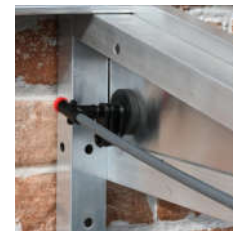
Inlet and link pipe
