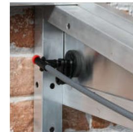
Inlet and link pipe
