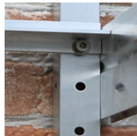
Bolt sits below staging rail
